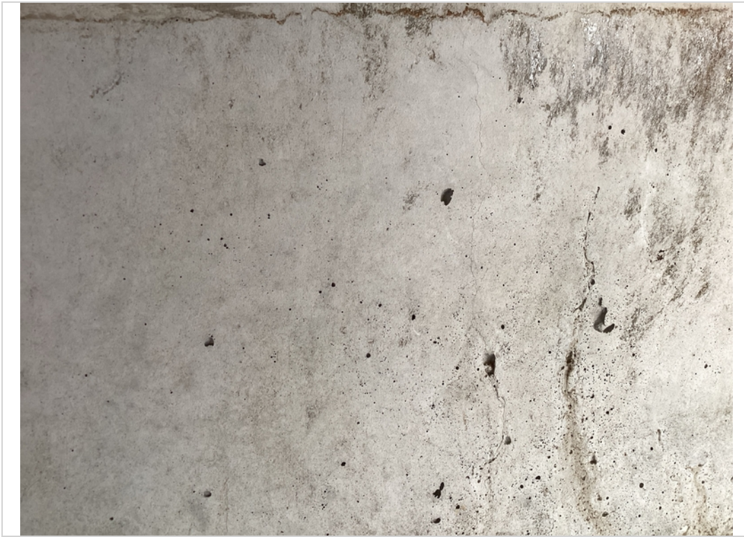
Span 1 slab H, hairline cracks
