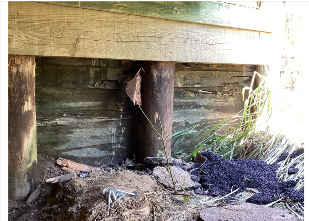
Breast wall at abutment 2 decay
