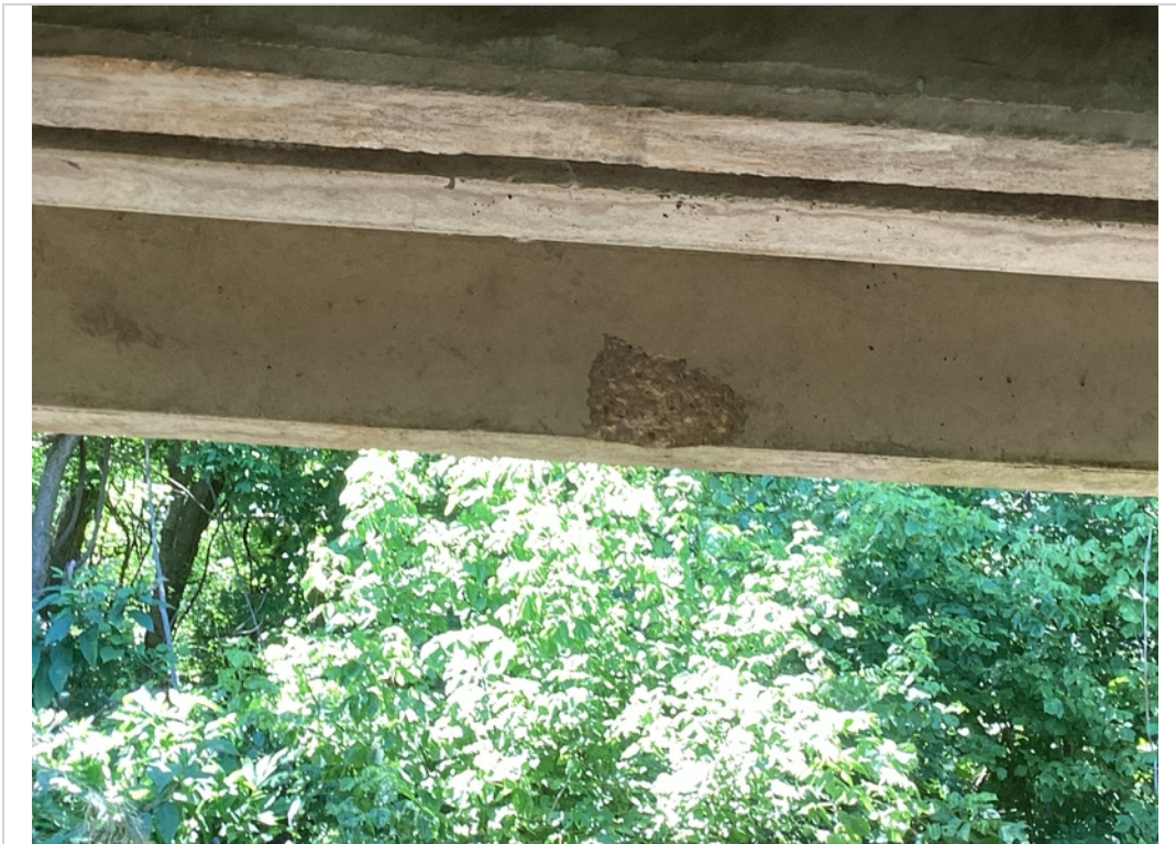
Span 1 slab A, damage
